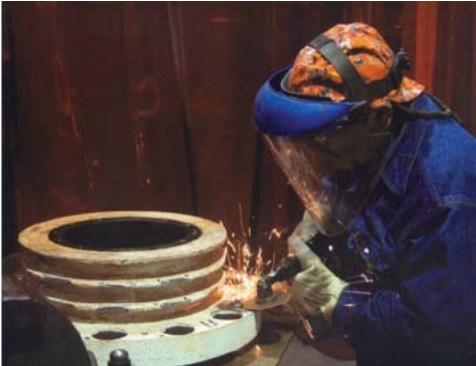
Photo by Local 1245 member Jim Zimmerlin captures welding work at PG&E's Diablo Canyon Power Plant.
