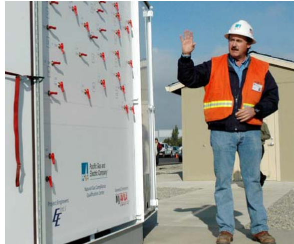
Senior Instructor Luis Faria shows off panel controlling gas flows to various training center locations.
