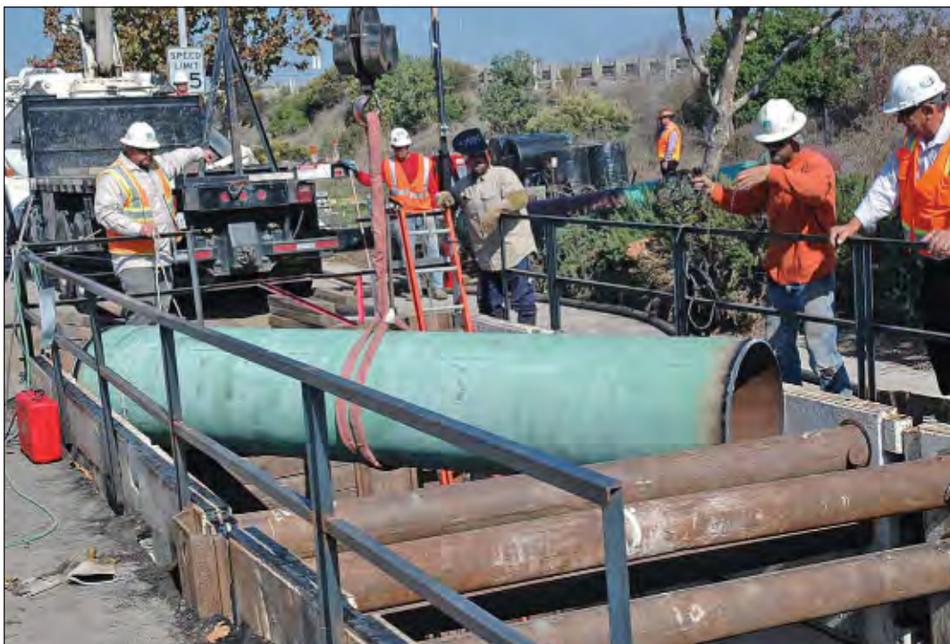
The pipe is carefully maneuvered into the narrow space through which it will be lowered into the vault.
