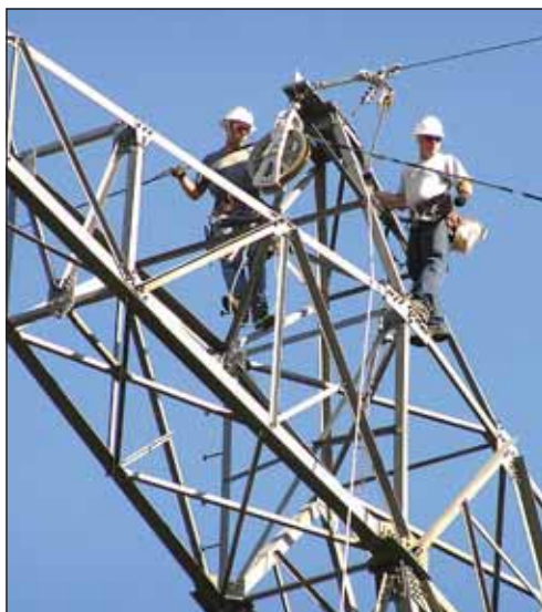
Apprentices Chad Rocco and James Clark get the anti-rotation device ready for the fiber.
