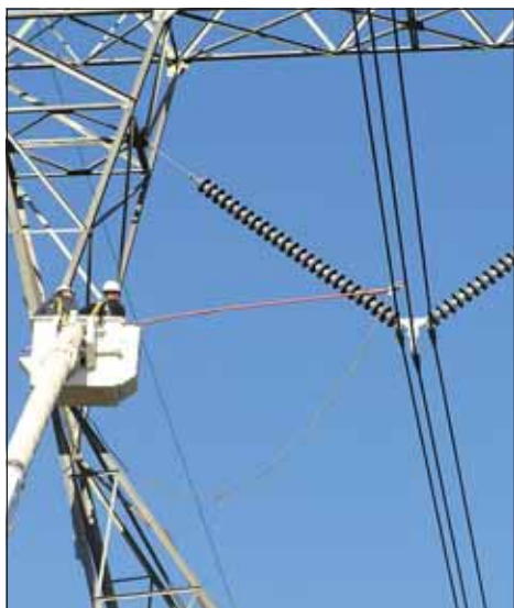
Lineman Dana Trimble and Chad Rocco ground the center phase of the Captain Jack / Olinda 500 KV line prior to fiber installation.
