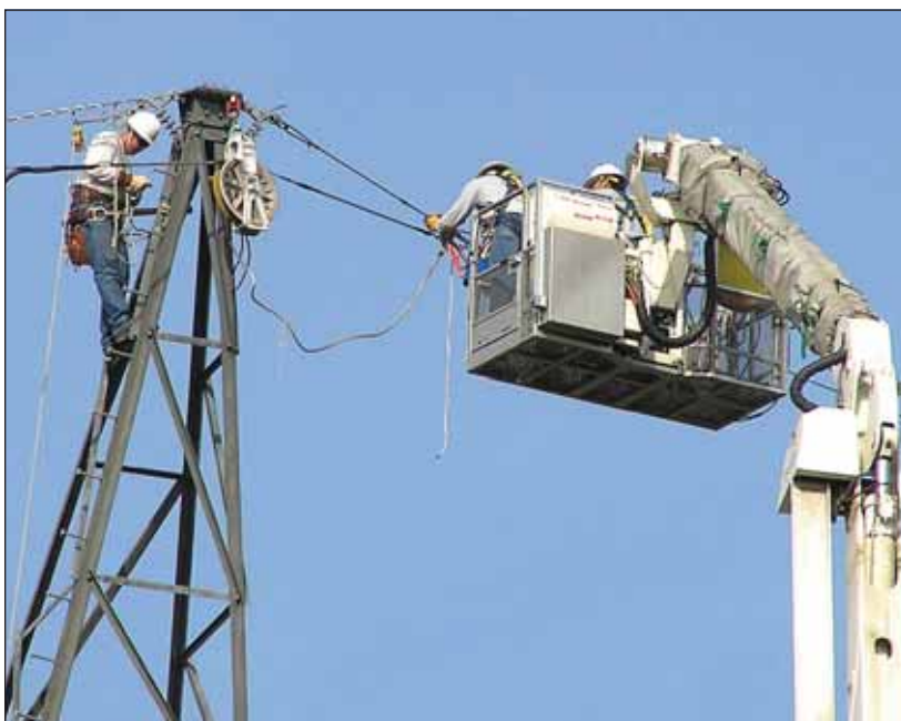
Lineman Joel Carrillo, James Hill and Apprentice Lineman James Clark remove rigging from existing static which was used to pull in the new fiber.
