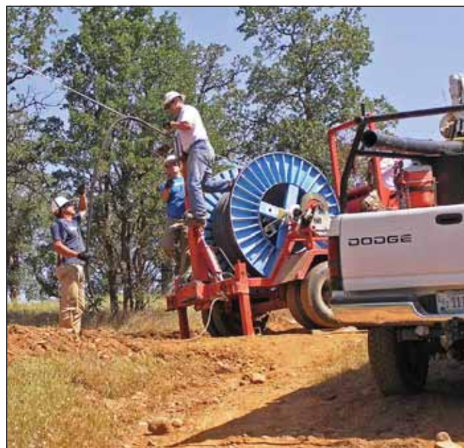
Linemen Darren New, Ryan Yeager and Apprentice Ryan Wheeler working at the puller.
