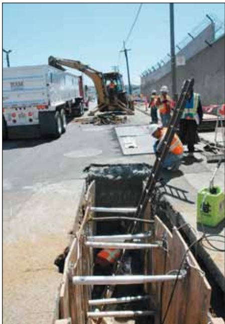
(ABOVE AND BELOW) Dirt from the trenching will be hauled away and disposed of by a contractor.
