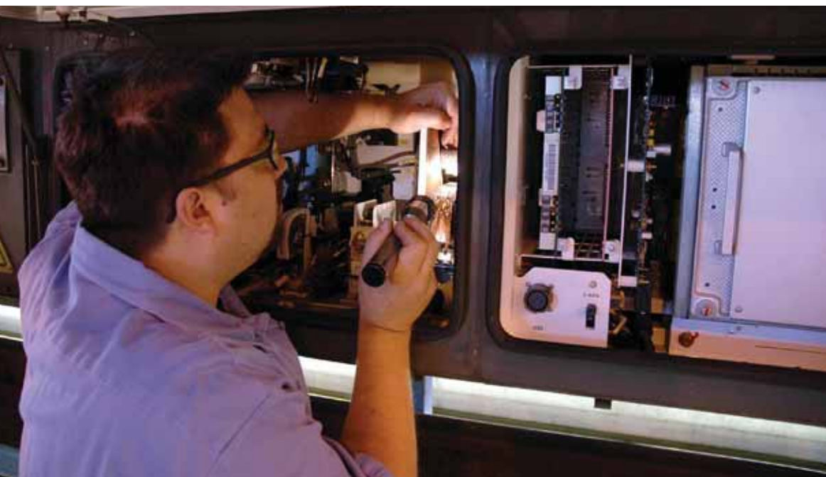
Brian Medeiros, an "A" Mechanic, inspects the main contactor for the LRV's propulsion system.
