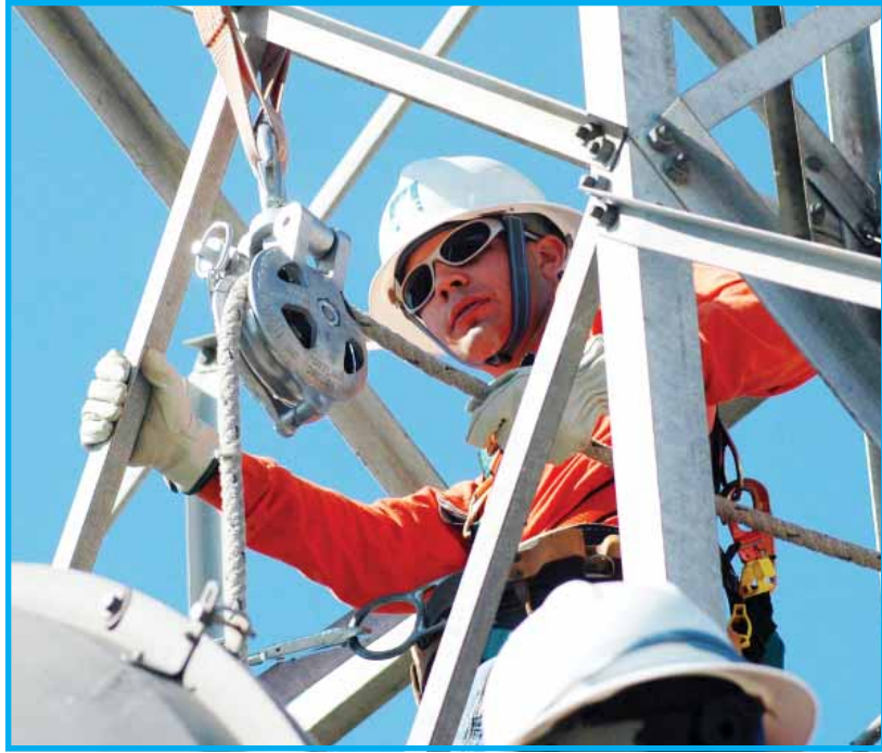
Travis Bess has just finished setting the load line for the dish removal.
