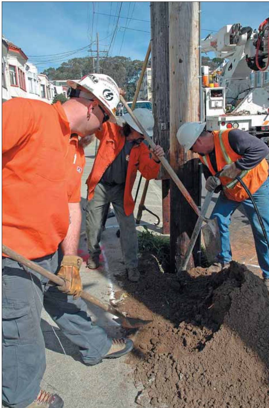
Packing fill around the base of the pole are, from left: Casey Kelly and Marshall Free, shoveling dirt, and Donald Mathews running hydraulic tap.
