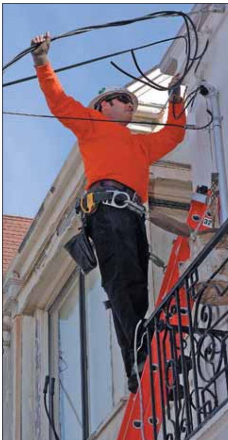
Jason Clause attaching new service to a house and making the weatherhead connections.
