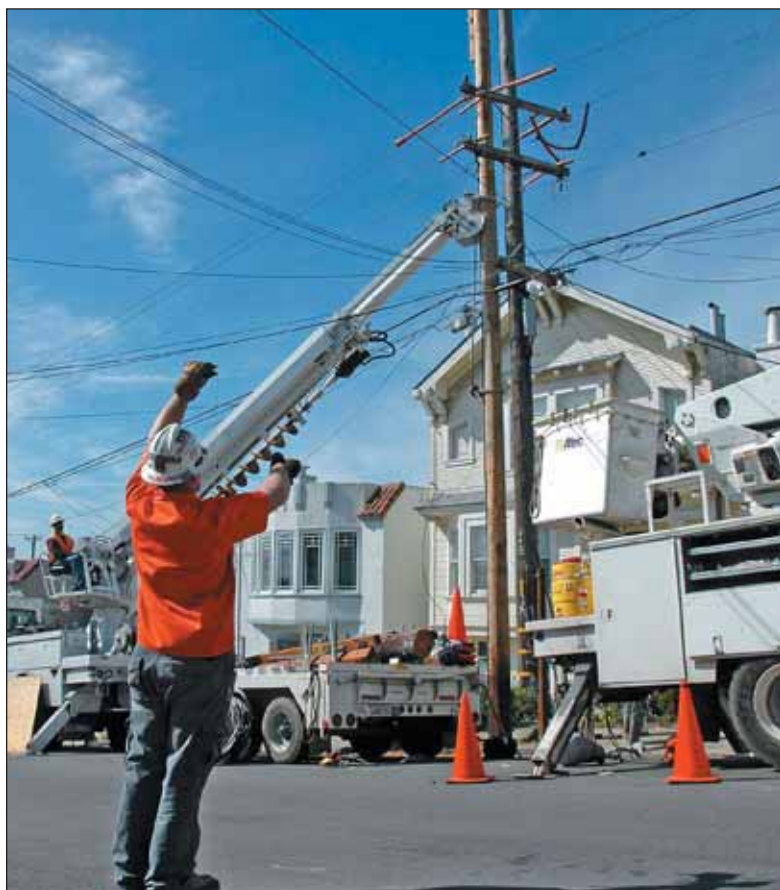
Casey Kelly uses a plumb line to make sure the new pole is level.
