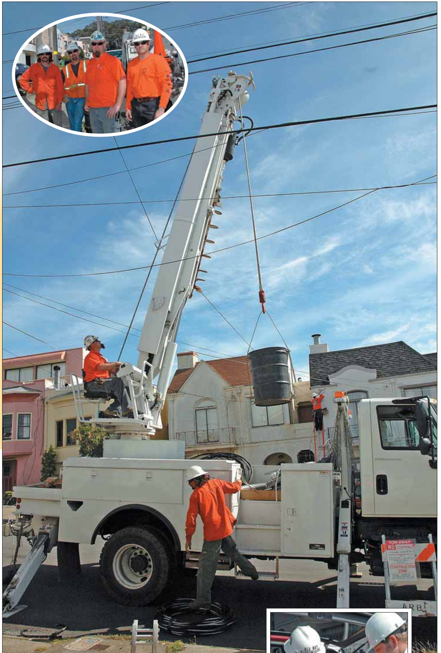
Casey Kelly picks up a bucket of fill to pack around the newly-set pole.
