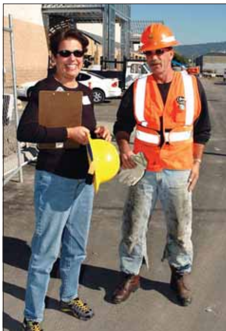
Local 1245 Business Rep. Lynne Morel and Lineman Gary Fenton talk shop in front of the new mall that will be served by the transformer being installed by the AP&T crew.
