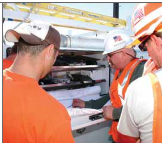
Line Working Supervisor John Deschaine reviews the situation with (from left, Ken Swain (obscured), Erik Rivera and Michael Stofer.
